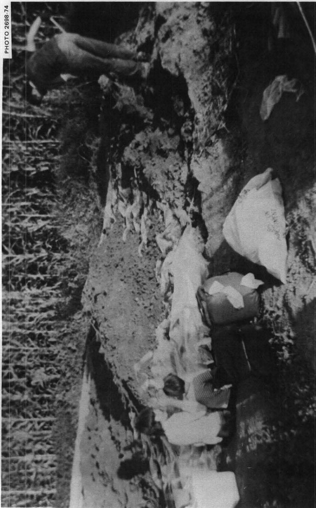
Fig. 4.9. Shoveling earth onto the "buried roof" made of a large piece of 4-mil polyethylene. After earth had been mounded onto the roof logs until it was about 18 in. deep along the centerline, the polyethylene sheet was spread over the entire roof area.
